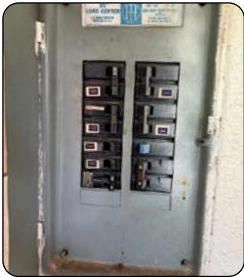
60 amp service panel is inadequate. Entire house would need to be rewired.
