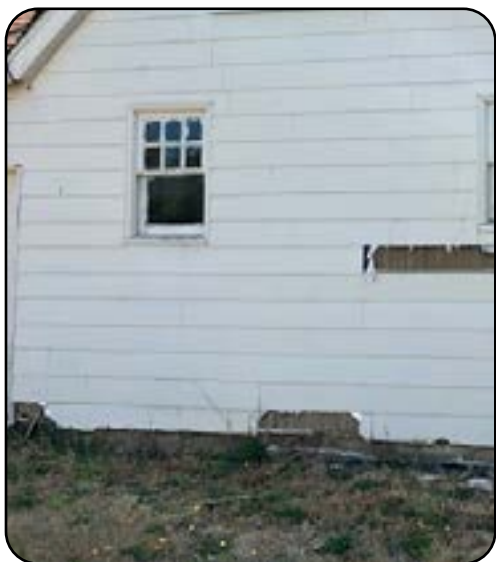
Failing asbestos siding. (back of the house sits on the ground with no foundation.)
