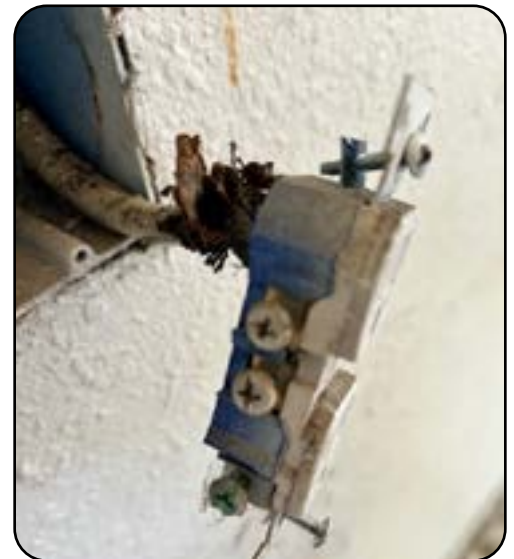
Wiring with no ground. Difficult to tell if it is 12- or 14-gauge.
