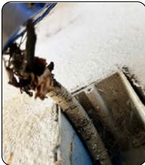
Cloth covered two-strand wiring without ground.
