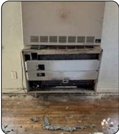
Outdated gas heater should be replaced. New heating and air conditioning would be needed.
