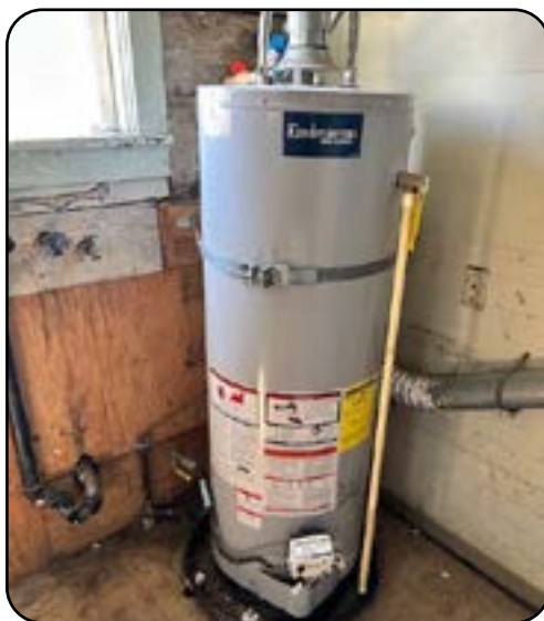
Gas water heater in questionable condition. (Dated 3.9.2016)
