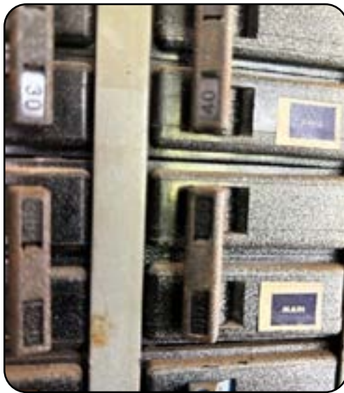
Dangerous electrical service would need to be completely replaced.
