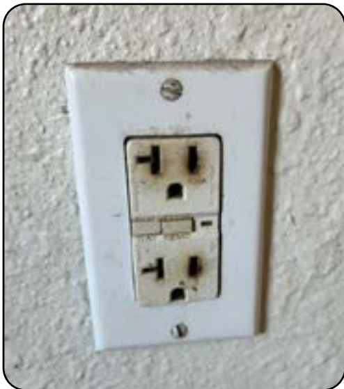
Arced and burnt GFI outlet.
