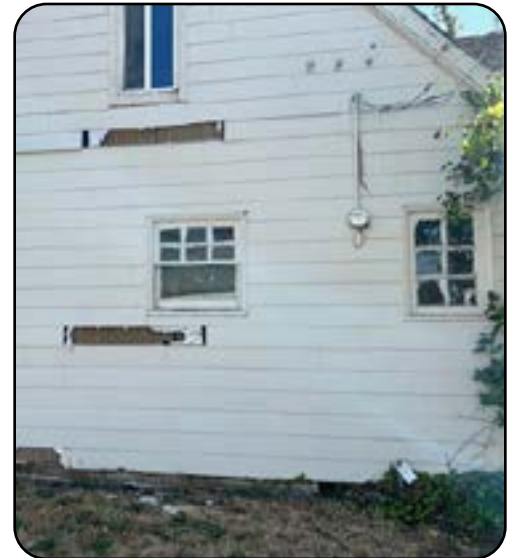
Asbestos siding failing. Broken pieces have fallen onto the ground. Several inefficient single pane windows would need to be replaced.
