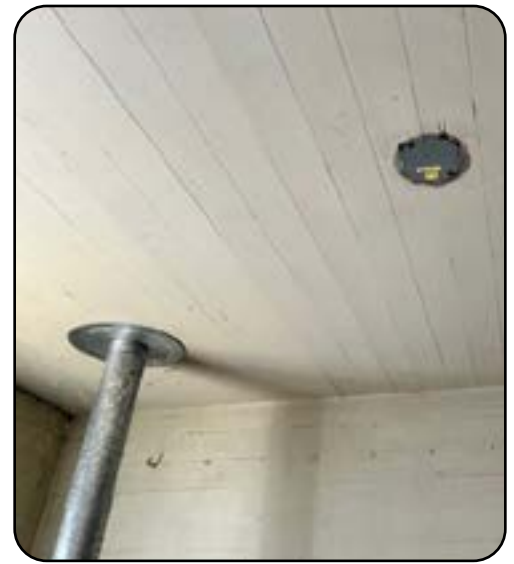
Utility room is not ADA compliant and has inadequate lighting.
