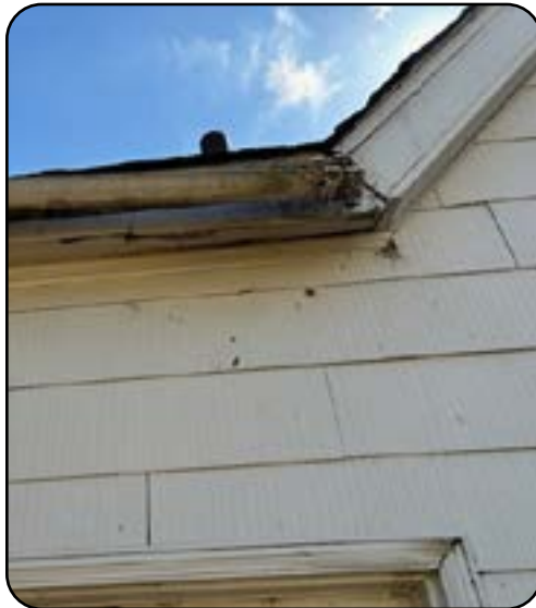
Failing gutters approximately 40-feet around the house. Gutters would need to be replaced.
