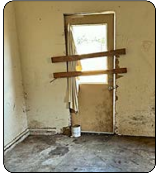
Backdoor would need to be replaced with a wider ADA compliant door.
